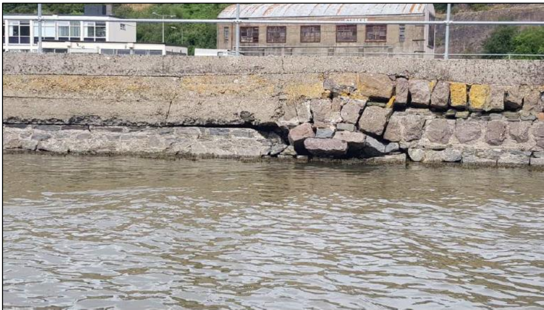
Plate 2.7 Defects on the existing quay wall – Dislodgement of blocks, mortar washout, several phases of wall upgrades (Ch. 550)
