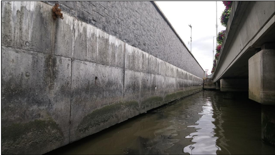
Plate 2.1 Typical condition of the wall/shoreline between Ch.0.0 and Ch.340 (photo taken at approx. Ch.200)
