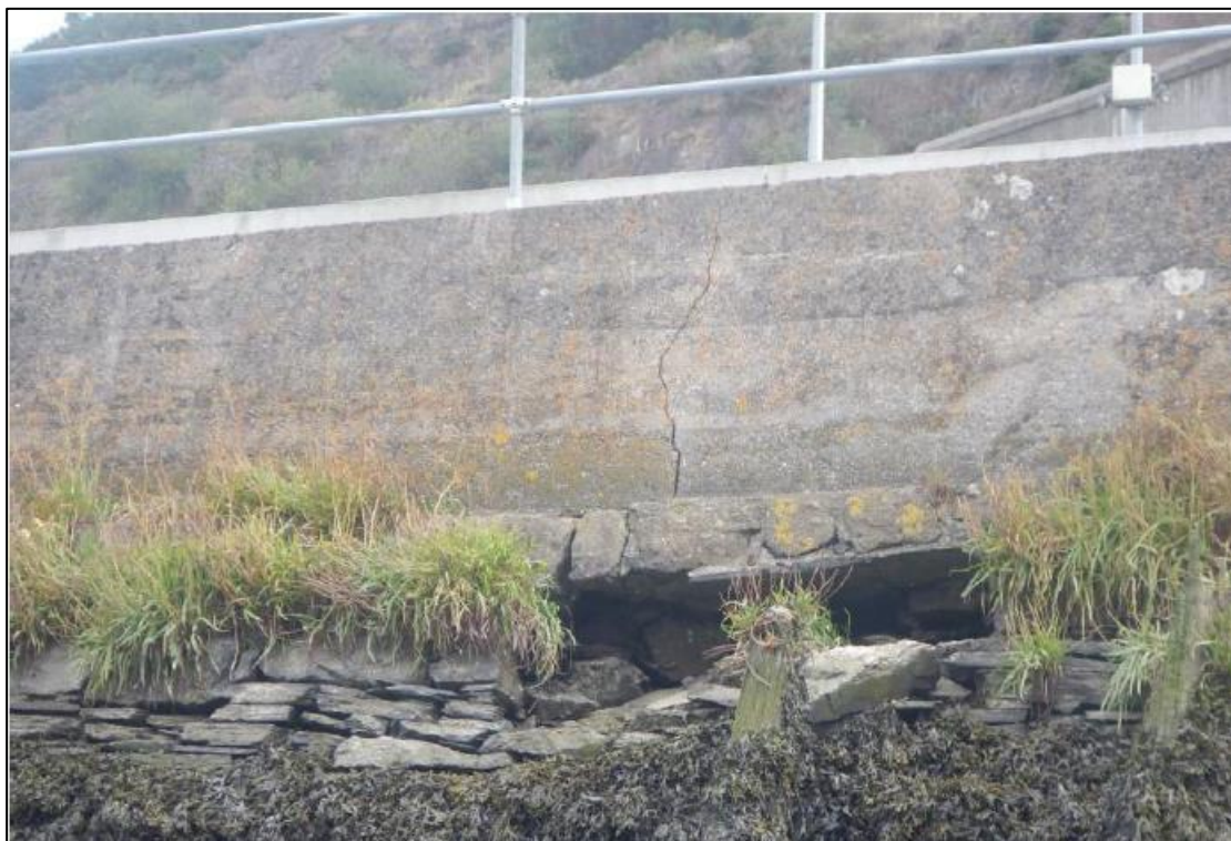
Plate 2.5 Defects on the existing quay wall – cracking of the wall and dislodgement of masonry blocks (Ch. 370)
