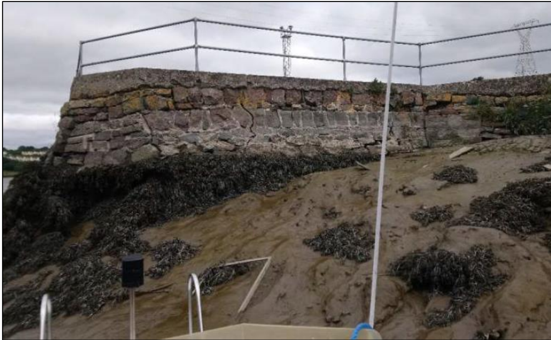
Plate 2.6 Defects on the existing quay wall – large displacement and rotation of the wall (Ch. 540)
